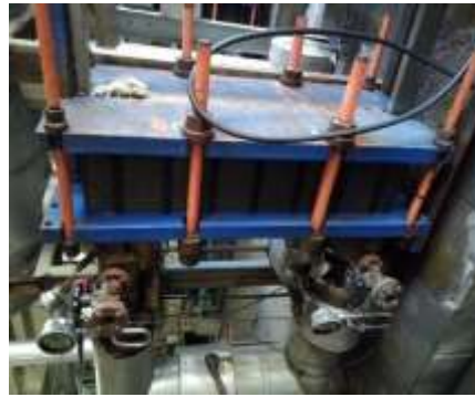
Figure 3: Plate Heat Exchanger at MRSDMM
