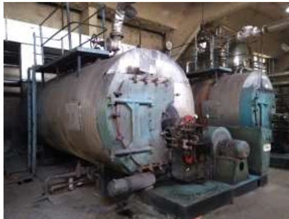
Figure 1: Fire tube boiler at MRSDMM
