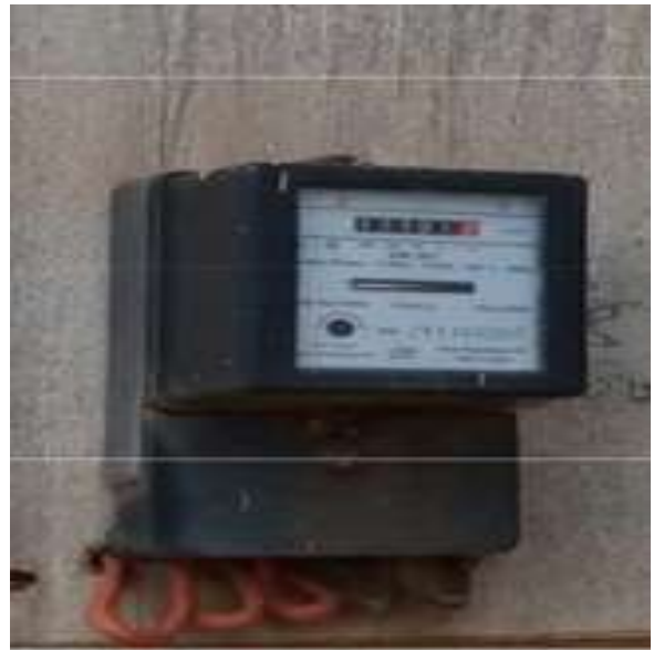
Fig.2. Electromechanical energy meters track power use.
