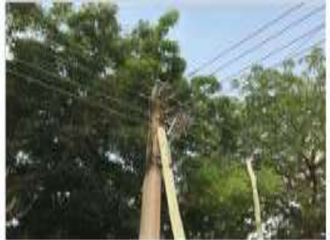
Fig. 1. Cable for service distribution.
