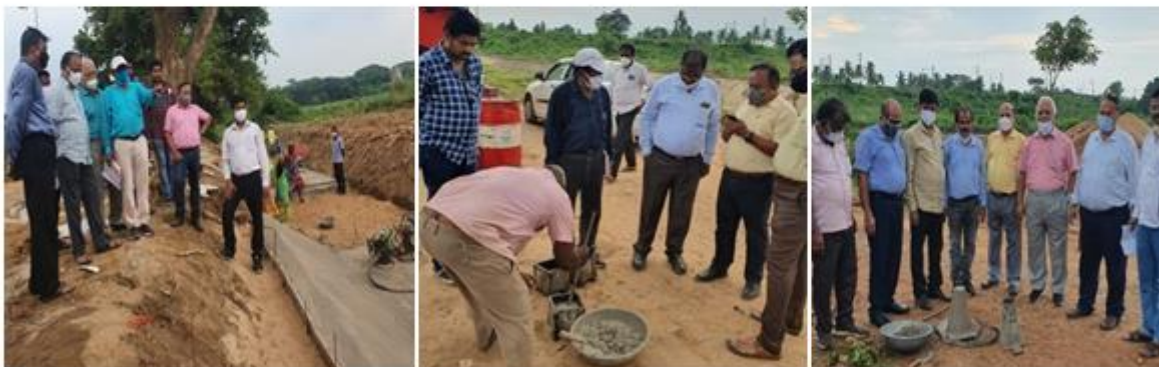
Fig.5 Pictures at the time of casting of canal lining cube making, slump cone testing
