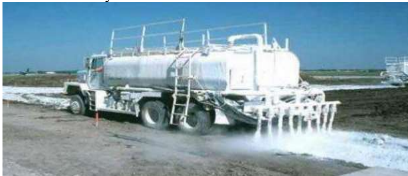
Figure 2: Shows the spreading mechanism of lime over the bed layer of soil.
