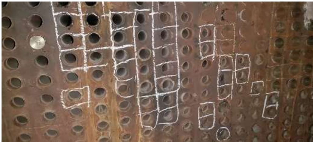
Fig. 2. Air preheater inside damaged tube (White marked)
