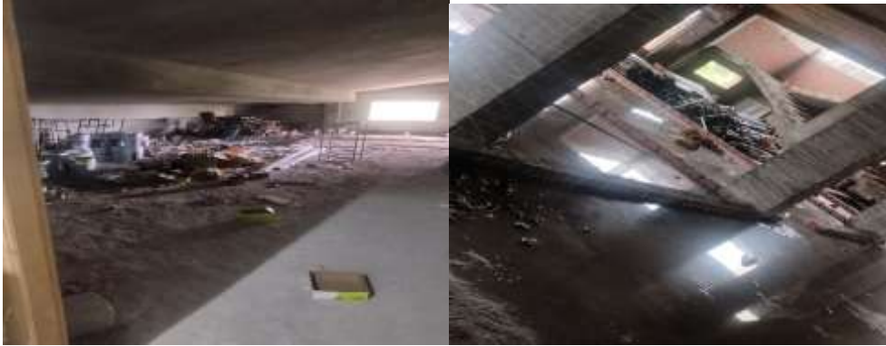
Fig (b) contaminated and hazardous waste
