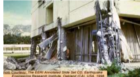
(a) 1971 San Fernando Earthquake
