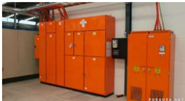
Fig. 10. Automatic power factor correction unit separate from main switchboard.
