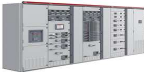
Fig. 9. Automatic power factor correction unit inside the main switchboard.
