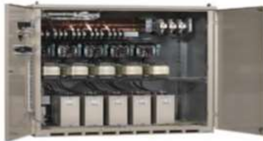
Fig. 4. three phase series reactors
