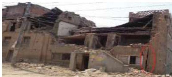
Figure 1-1: Brick Masonry Failures in Buildings
