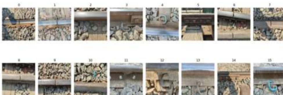
Figure 2: Tracks without Defects
