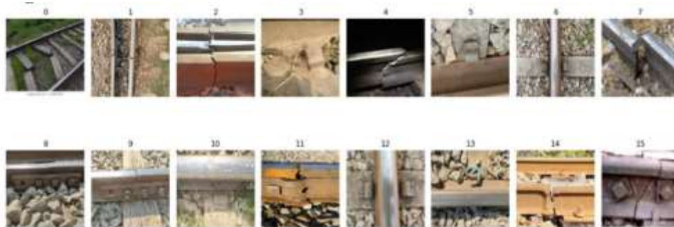
Figure 1: Tracks with Defects
