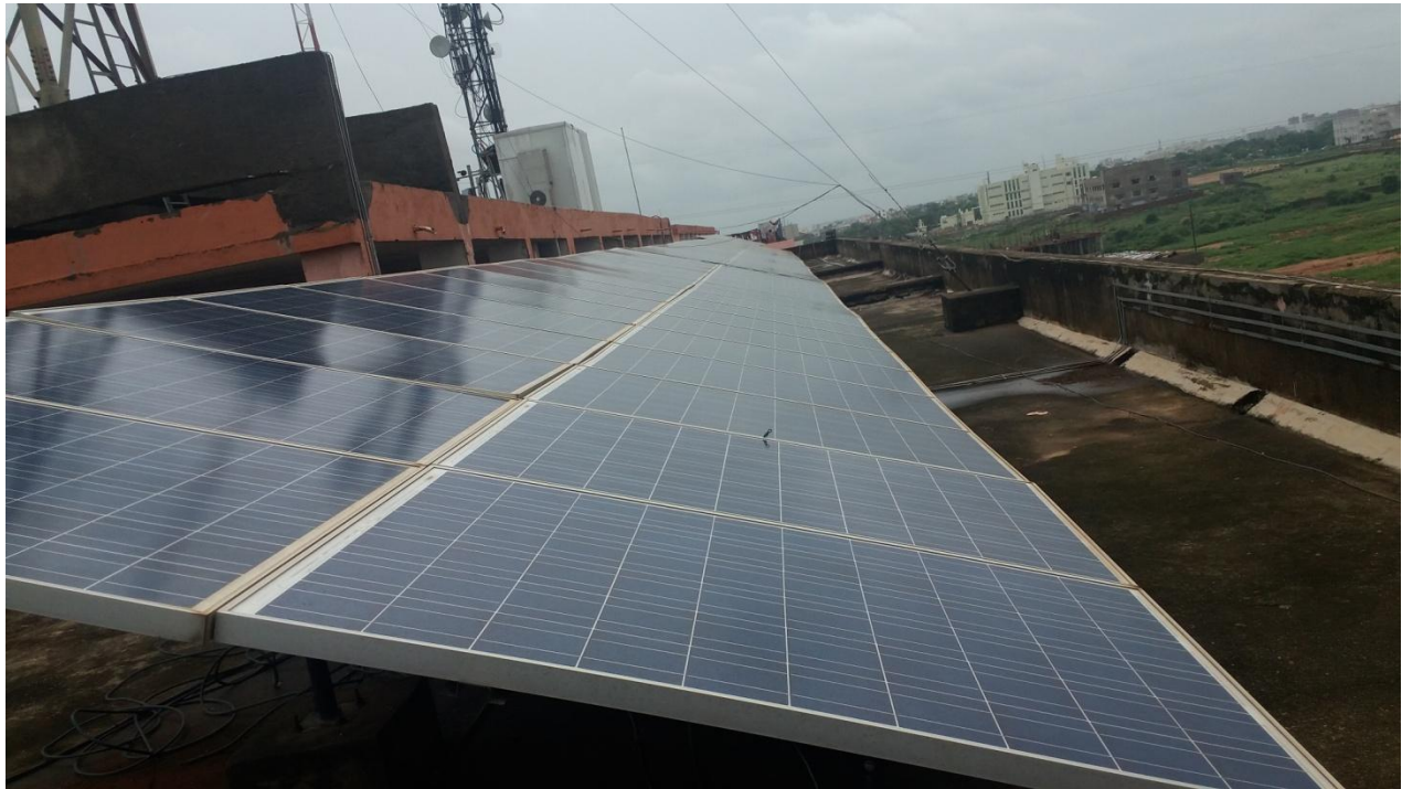
Figure 2: 50kW p roof top PV system of KIIT
