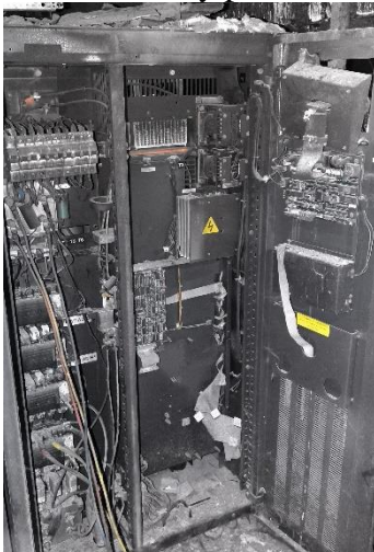
Figure 2: Burned out UPS
