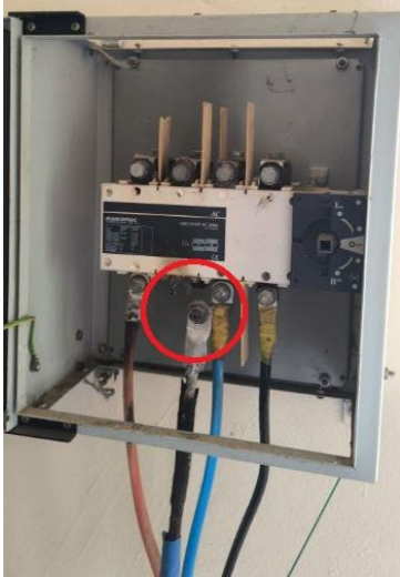
Figure 3: Damaged Phase due to Overload
