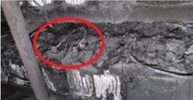
Figure 1: Batteries which has completely burned
