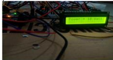
Figure 43: Output of Power from the Solar Tracker under High Light Condition.
