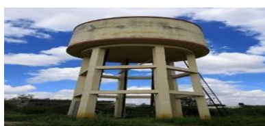
Fig – 1 – water tank
